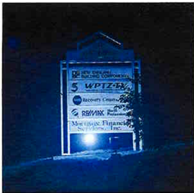
Sign lights should be carefully located and aimed to prevent glare. (PHOTO: GARY CLAYTON HALL)
